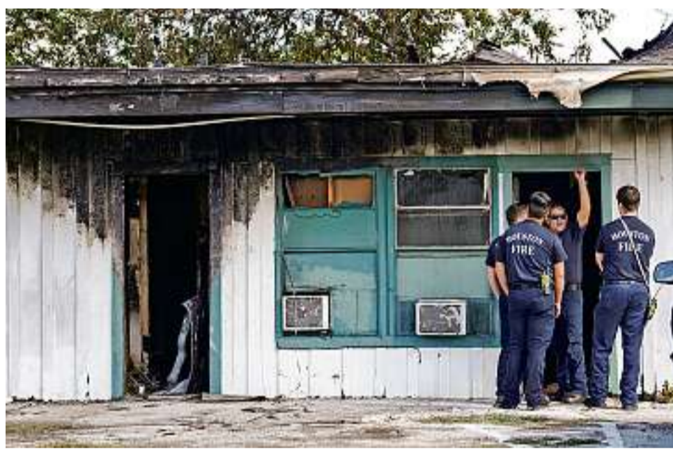
Firefighters at a burned building in Houston where fleeing residents were shot and killed on Sunday
