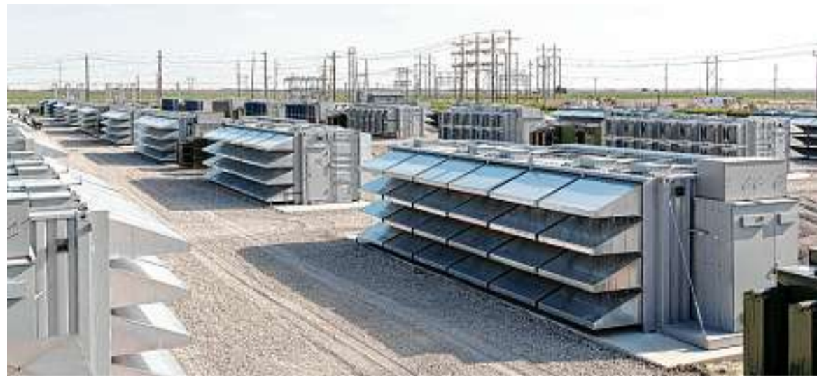
A Compute North data center in Kearney, Neb., shown last year.
