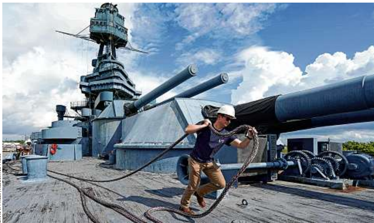
OLD WARRIOR: The Battleship Texas, which was commissioned in 1914 and served in World War I and World War II, is scheduled to be towed down the Houston Ship Channel on Wednesday to a dry dock in Galveston. Once there, it will undergo a $35 million repair.
