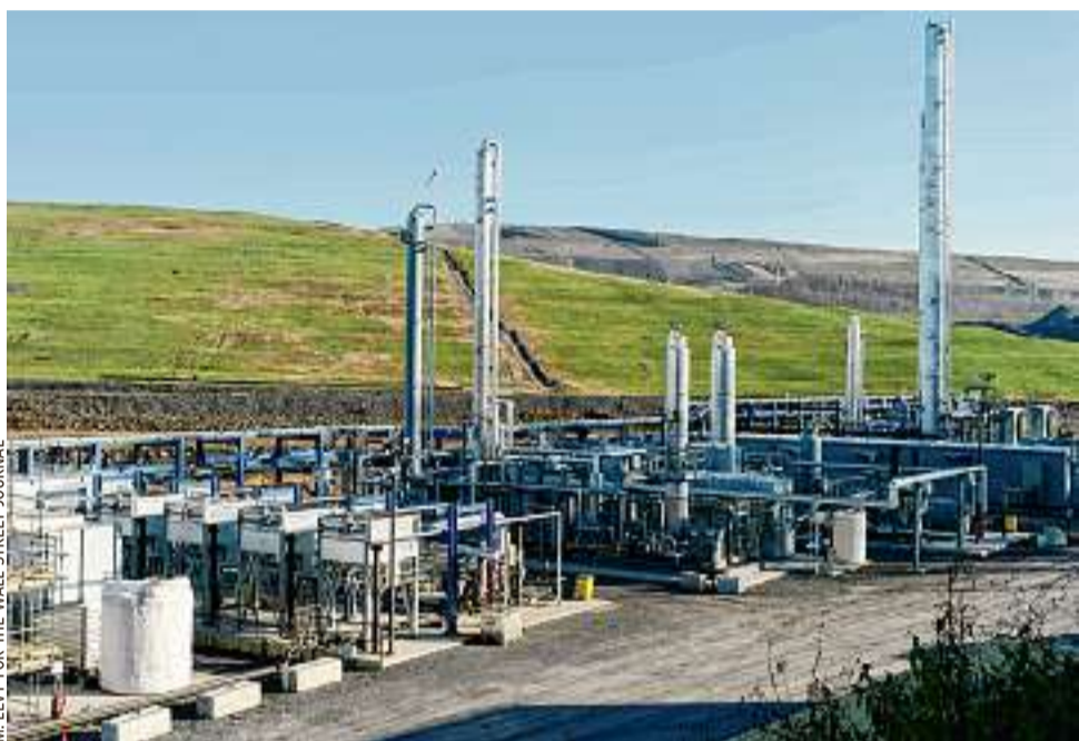
An overview of the Project Assai, built by Archæa Energy, at the Keystone Sanitary Landfill
