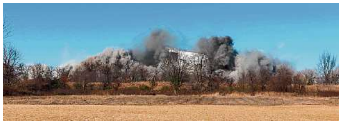
Smoke and dust rose from the site of a former coal-fired power plant in Logan Township, N.J., after it collapsed when explosives were detonated to implode it on Friday. The facility was one of the last two coal plants in the state. Both closed three months ago.
