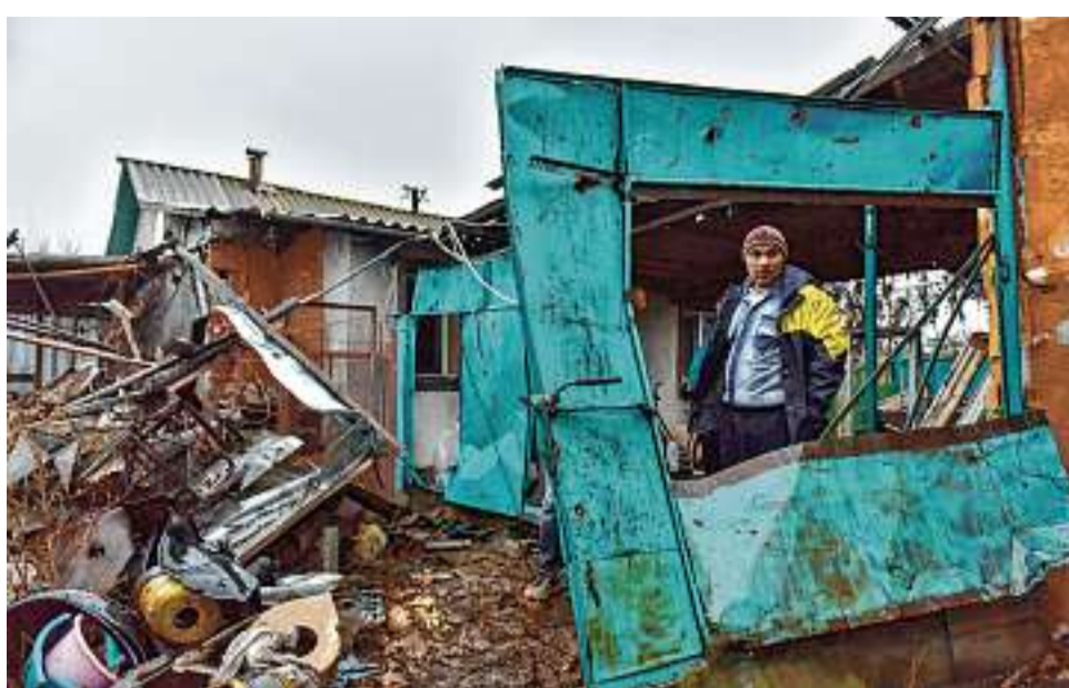
A resident returns to his damaged Shyroke village home in the Mykolaiv region of Ukraine.
