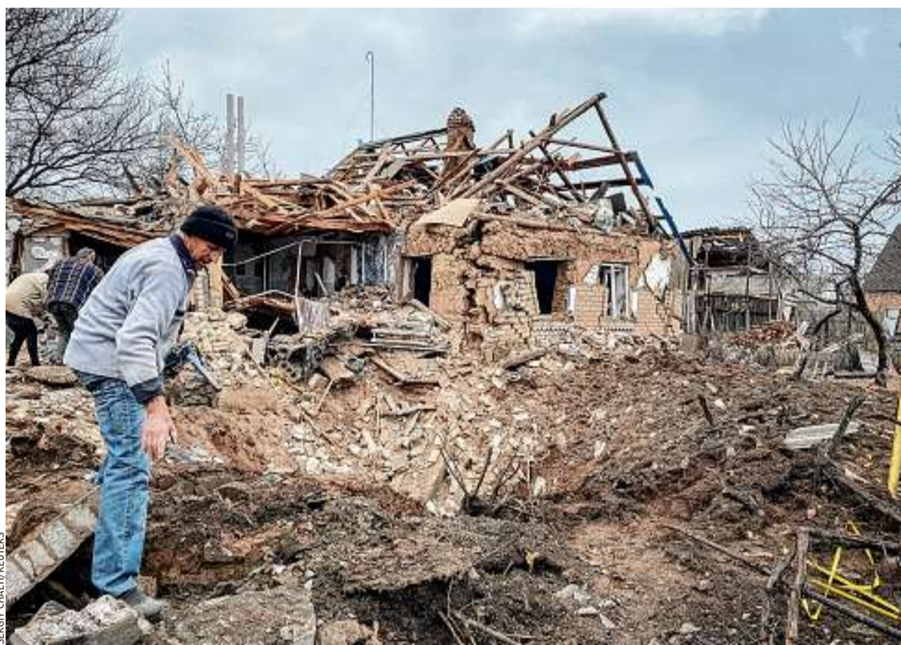
Residents inspected the damage on Monday after a Russian military strike in Ukraine's southeastern Zaporizhzhia region.
