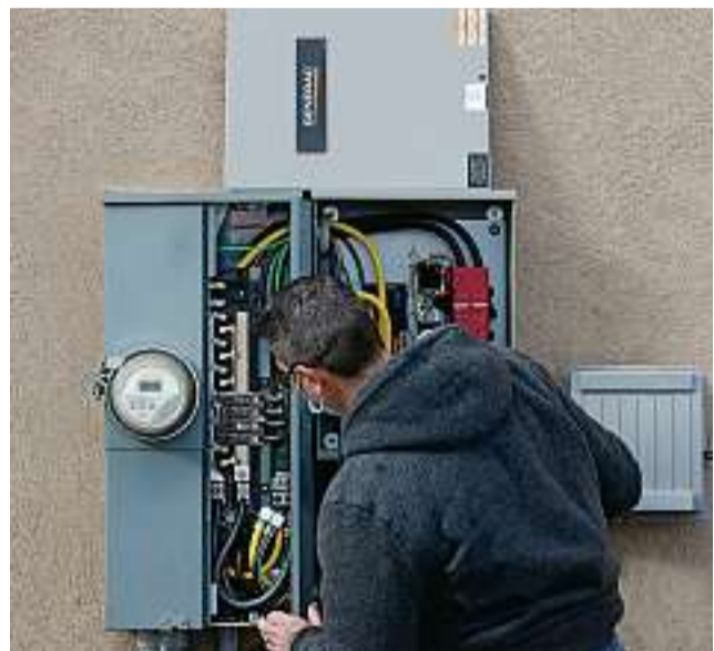
An electrician inspects a new power box for a Generac generator.
