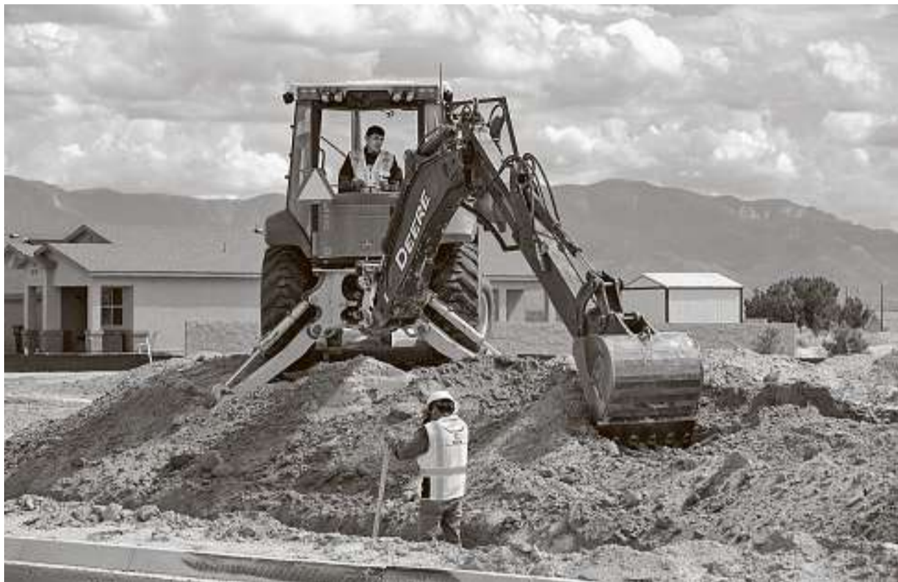
Workers install utilities at the site of a home being built in New Mexico. Utility stocks are known for their sizable dividends.
