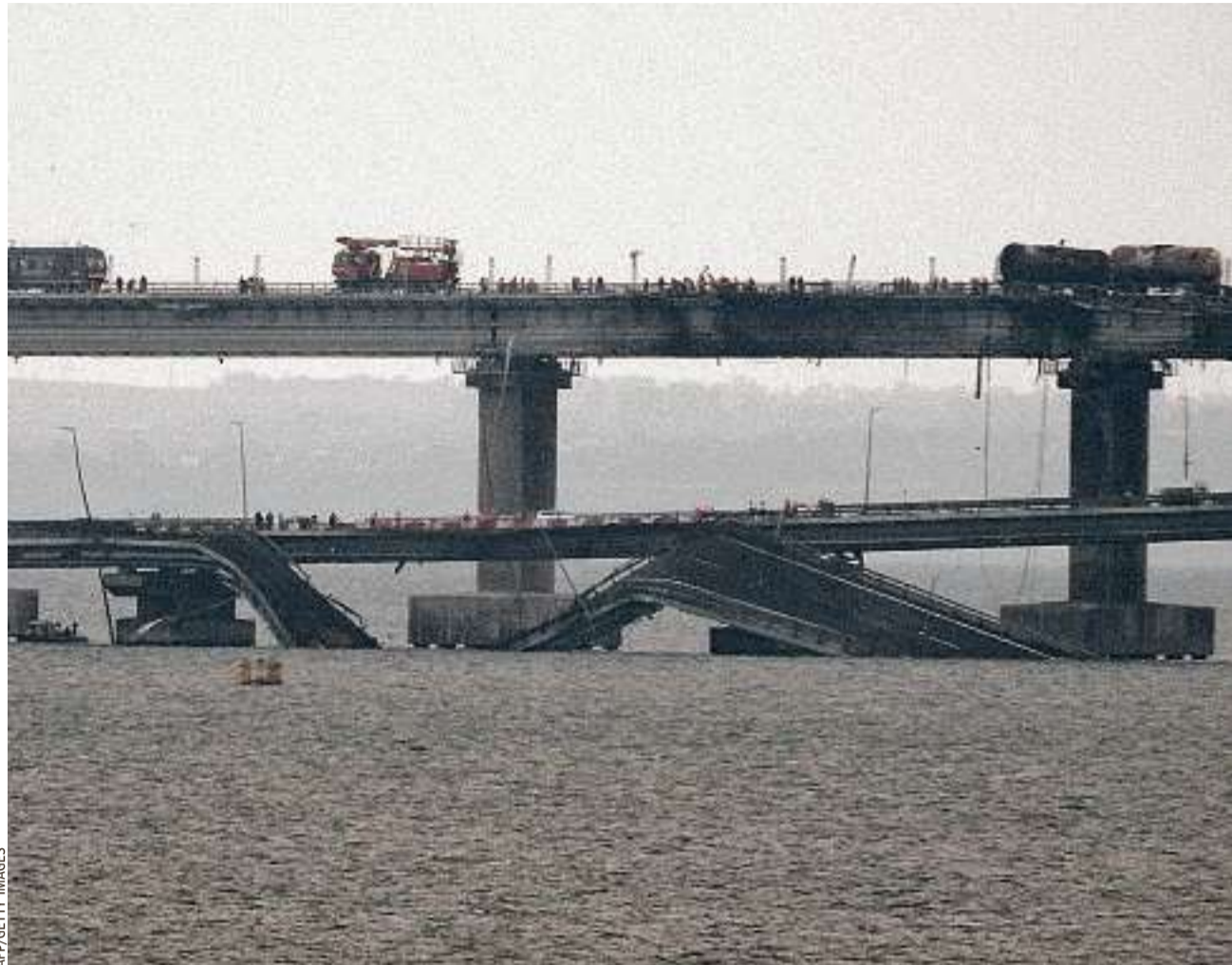
REPAIRS: Workers restored railway tracks Sunday on the Kerch bridge linking Crimea to Russia, a day after it was damaged by an explosion that Russia blamed on Ukraine. The damage could hurt Moscow's war effort in southern Ukraine. A7
